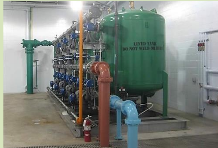
City of Reading Treatment Plant
