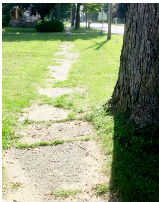
Existing sidewalk condition in need of repair.
