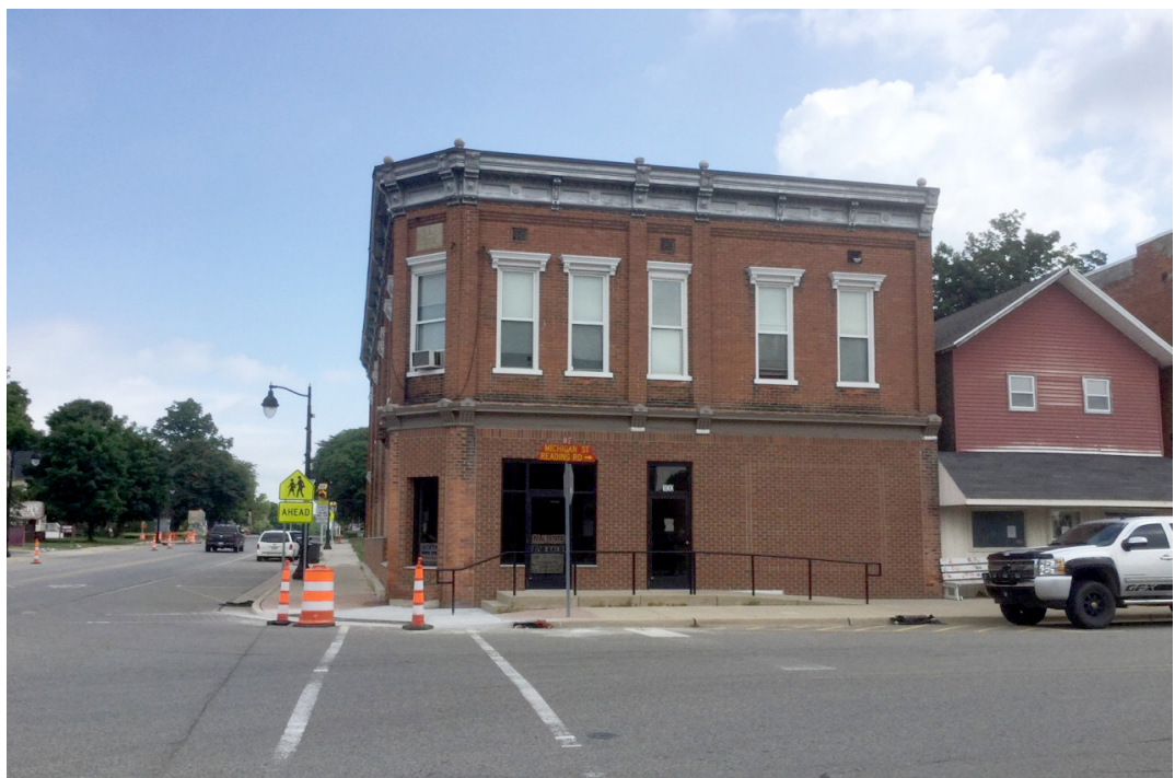
MEDC grant money used to rehabilitate rental units on the second floor.
