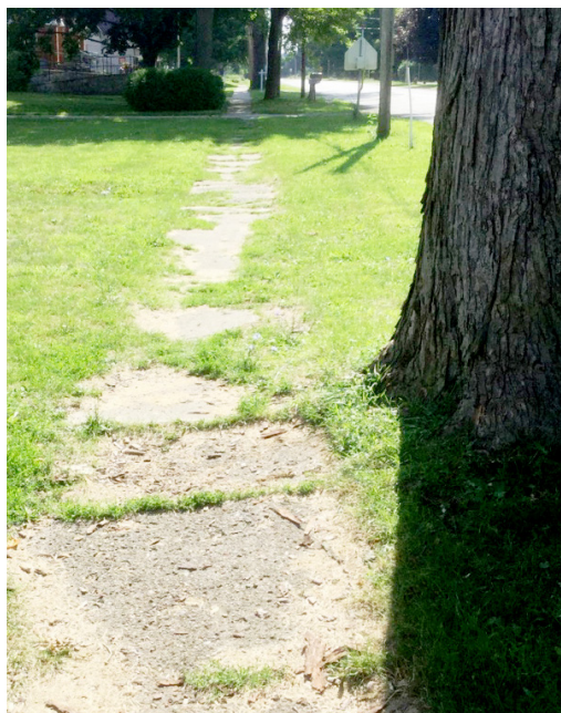
Existing sidewalk condition in need of repair.
