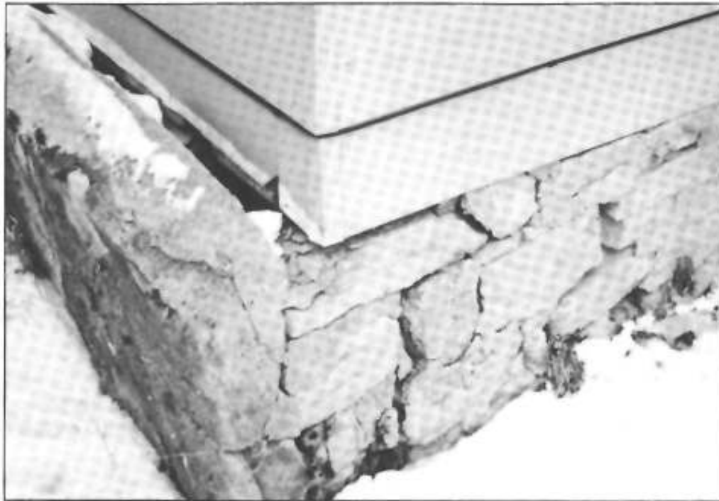
Commentary Figure 304.5 MAJOR DAMAGE TO A FOUNDATION WALL This foundation is crumbling. Failure to repair it will eventually lead to its collapse.
